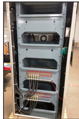
CUBE-BB48E2EV1 Back Panel Removed
