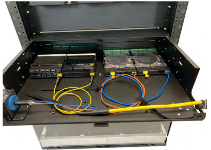
MTG MPO Riser Cable—Rear View
