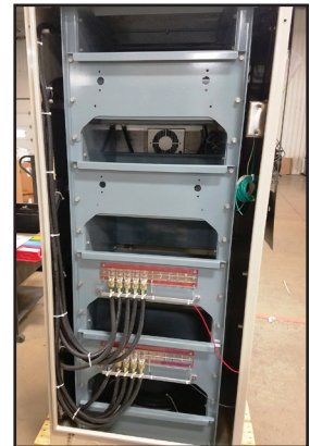
CUBE-BB48E2EV1 Back Panel Removed
