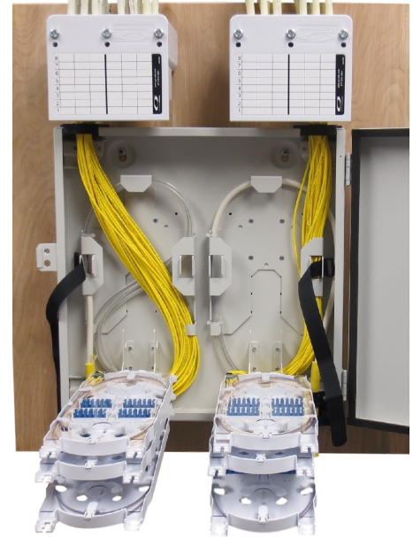
A: Fiber Splice Box (FSB) with Microduct Manifold
