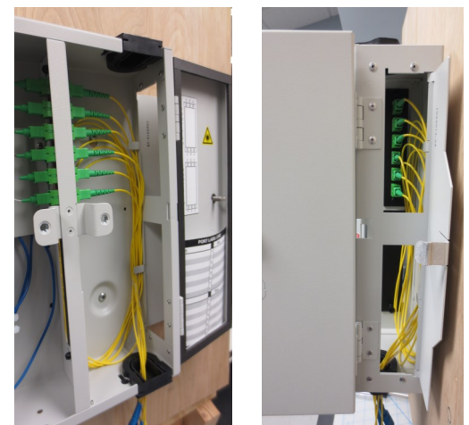
Inside Outside Access Door View
