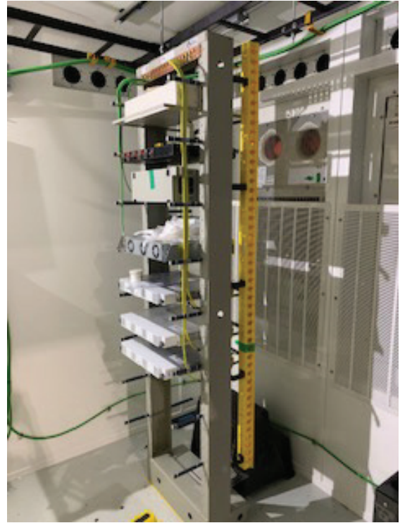
Interior View - Ericsson Racks
